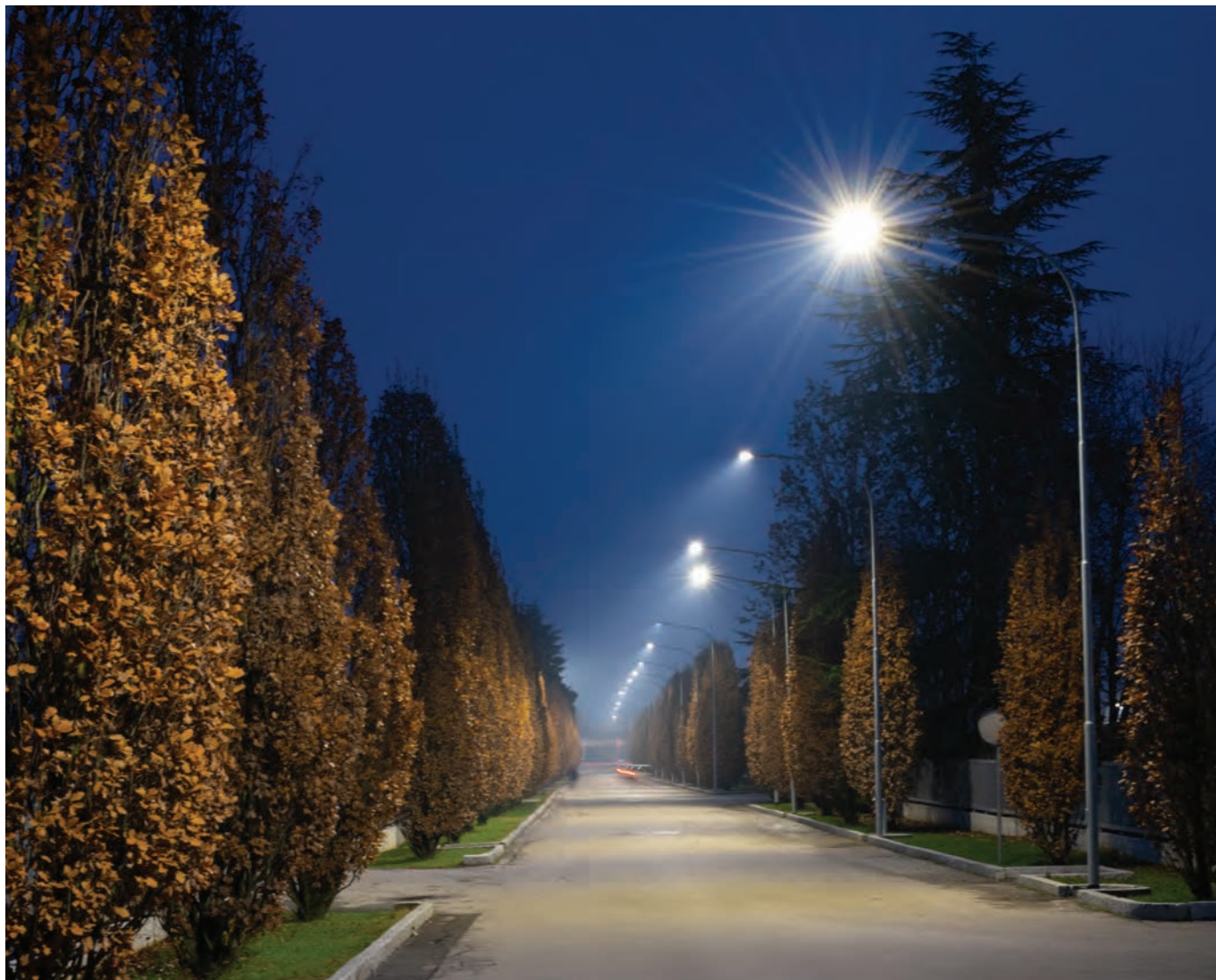
153 armature stradali / street lighting
